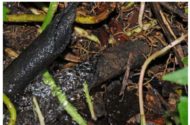
Damaged Soaker (Drip) Hose Gushing Water
